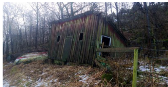
A construction barely holding together. Walls are sliding and roofs are gliding and the surfaces are turning color from moulds.
